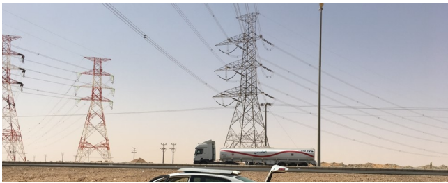
Fig. 3. Real oil truck crossing EHVAC transmission lines, 380 kV (Saudi Arabia).
