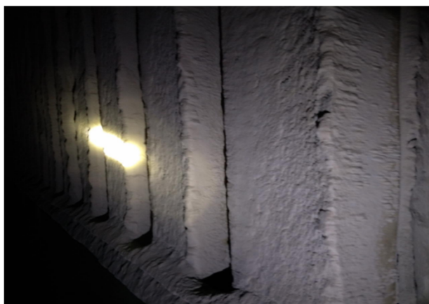
Fig. 1. Conventional groove plates and accumulated dust.
